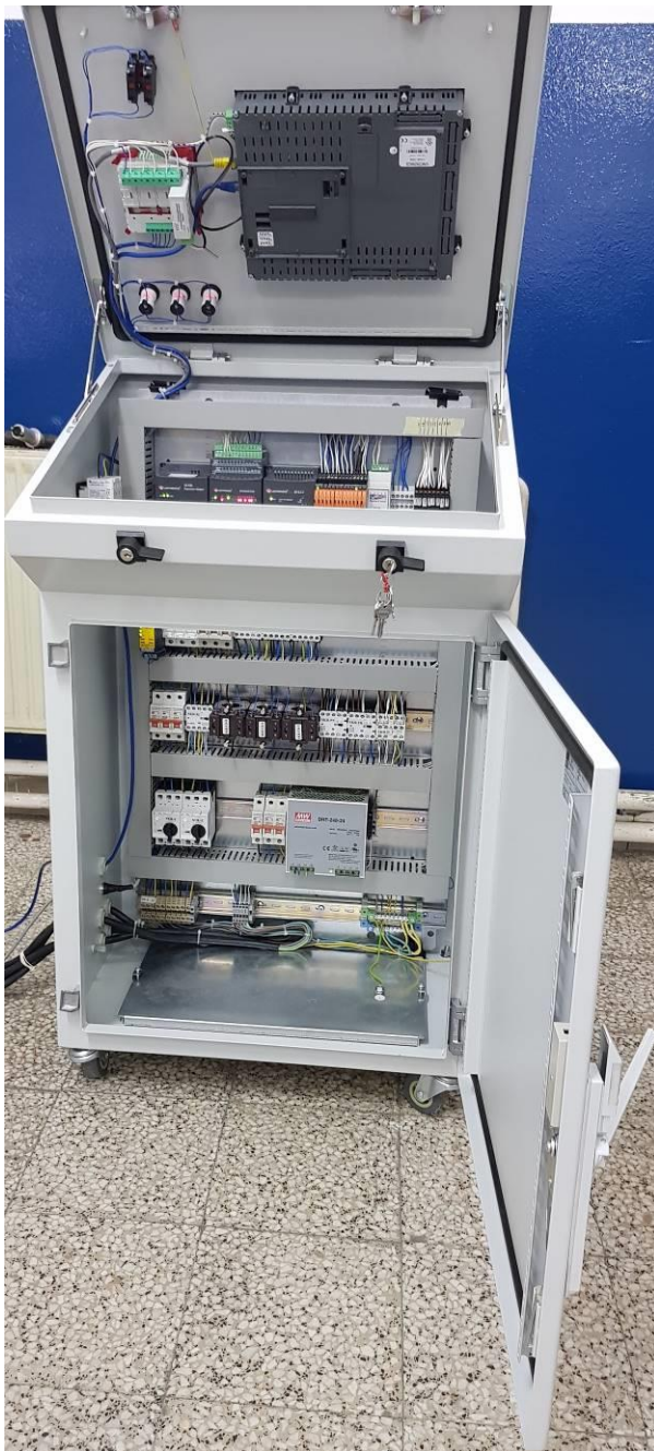
Fig.3. Arrangement of EPMFM equipment
