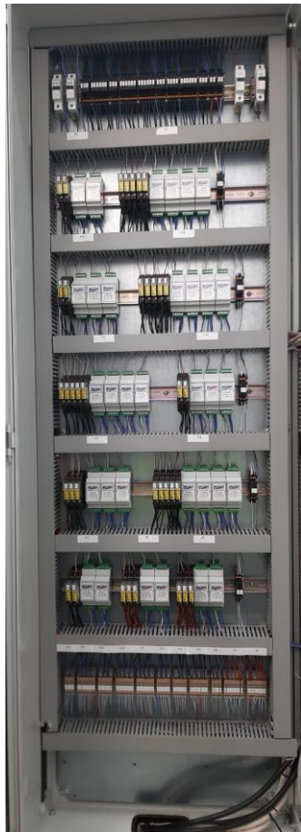
Fig.6. Cabinet with SM for Elemir EI
