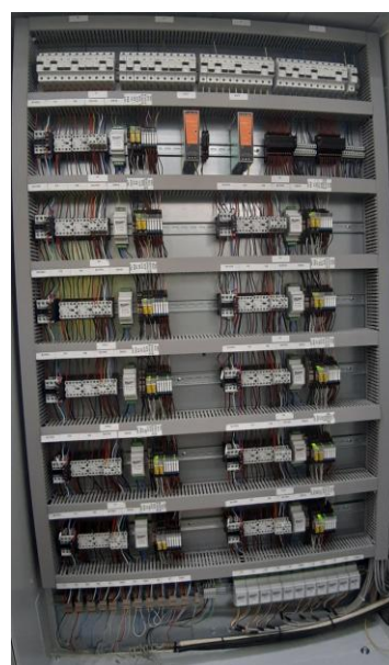
Fig.5. Cabinet with PM modules for Elemir EI
