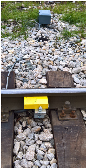
Fig. 2. EAC Outside Equipment
