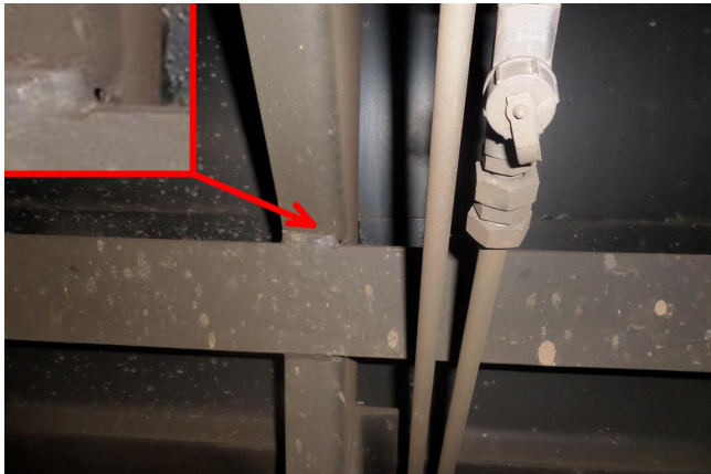
Fig.8. Crack in the welded joint on the actual wagon
