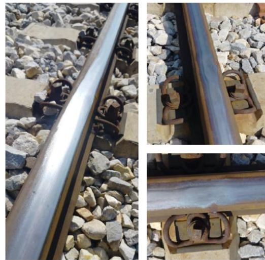
Fig. 5. Rail distortion caused by struggling train traction.
