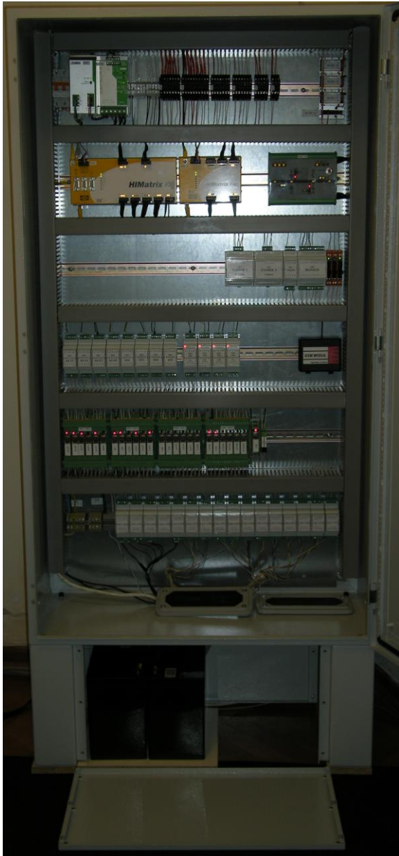
Fig.2. Controlling cabinet of the ELC system
