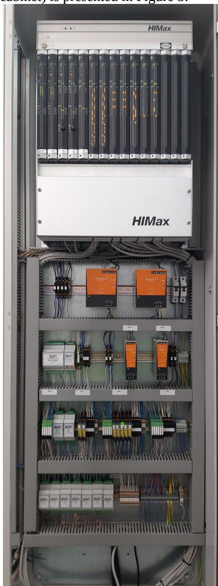
Fig.3. Central Safety Controlling System of Elemir EI
