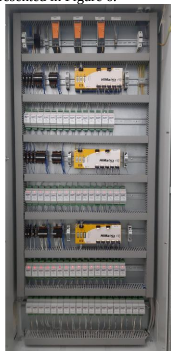
Fig.4. EAC based Train Detection system for Elemir
