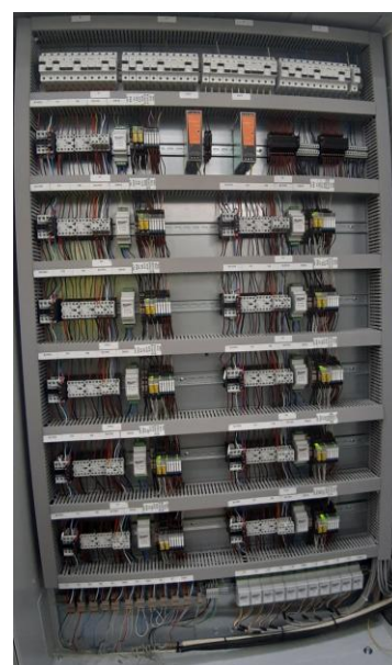
Fig.5. Cabinet with PM modules for Elemir EI
